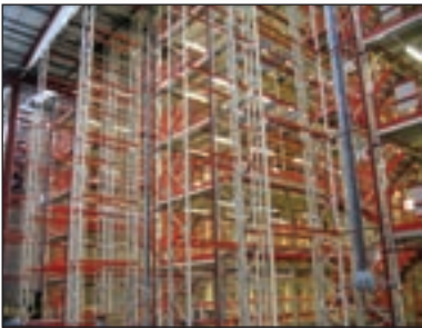
Picking floors constructed in between the pallet racking system
